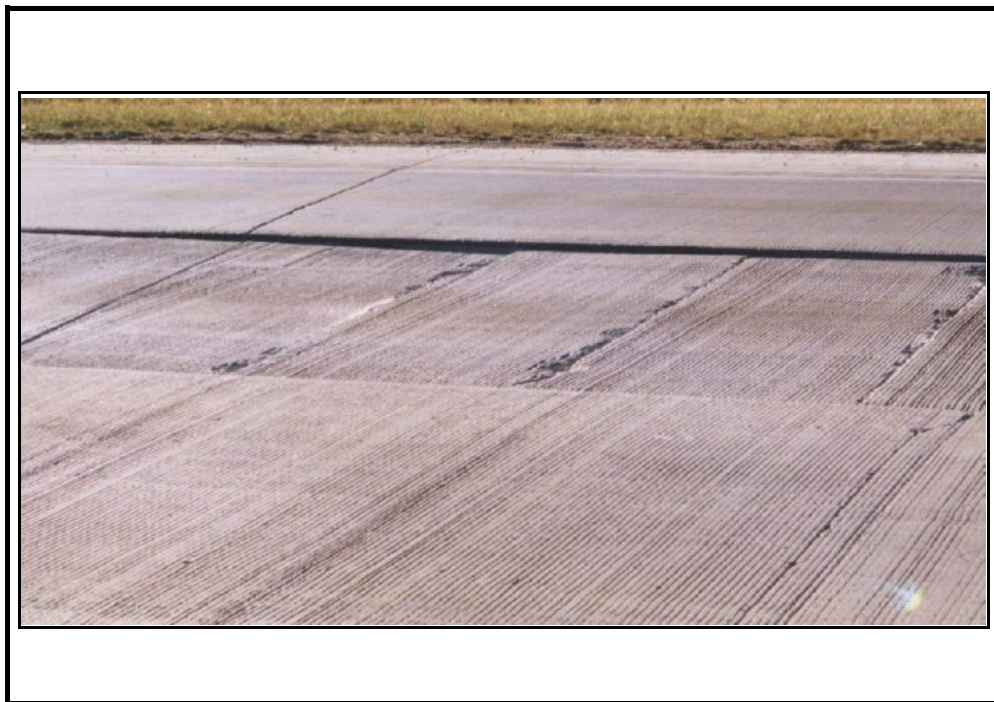
Photo C-11. Settlements in Jointed Concrete Pavement, Medium Severity
