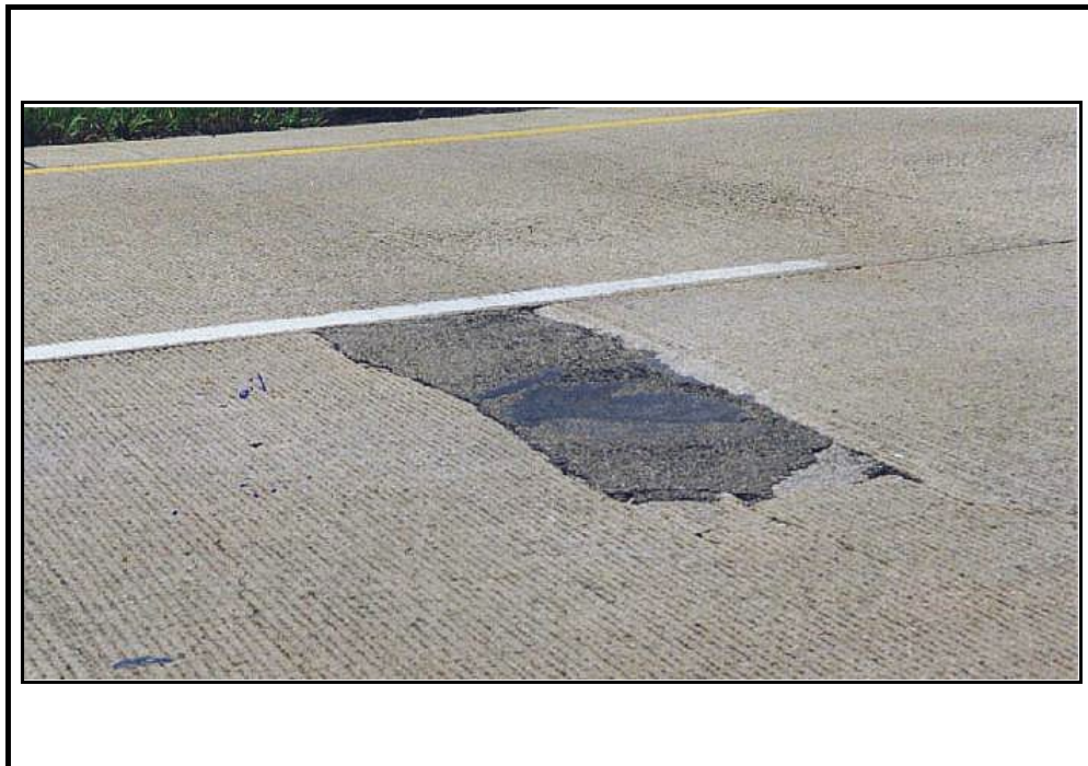
Photo C-6. Patching in Jointed Concrete Pavement, High Severity
