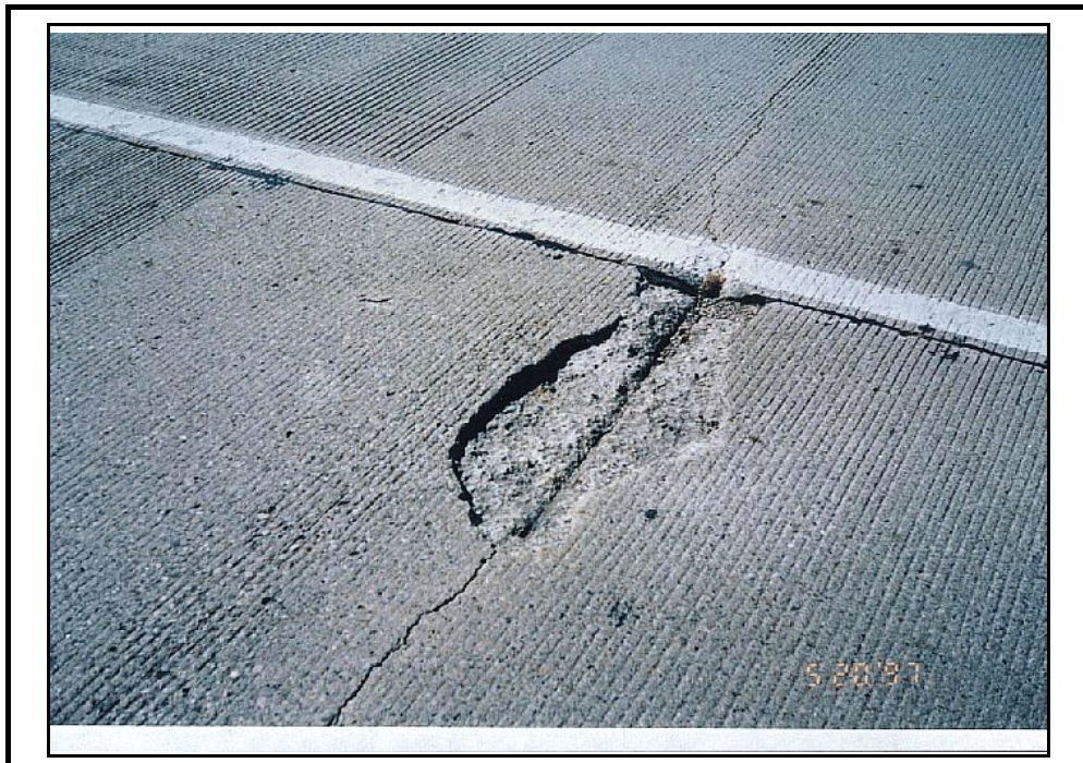
Photo C-17. Pressure Damage in Jointed Concrete Pavement
