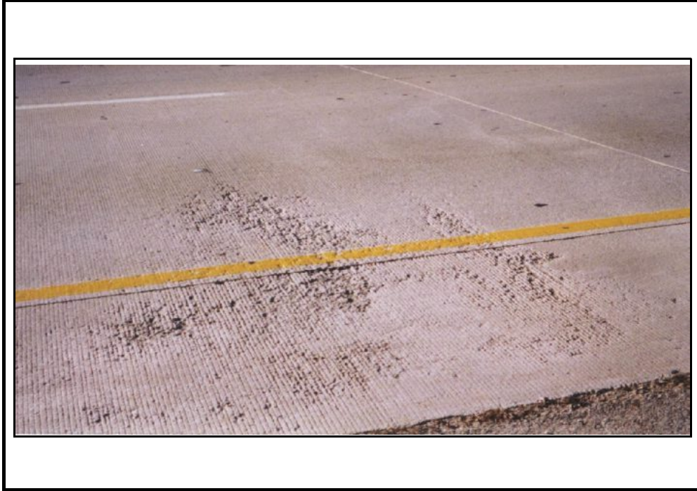
Photo C-1. Surface Deterioration in Jointed Concrete Pavement, Medium Severity
