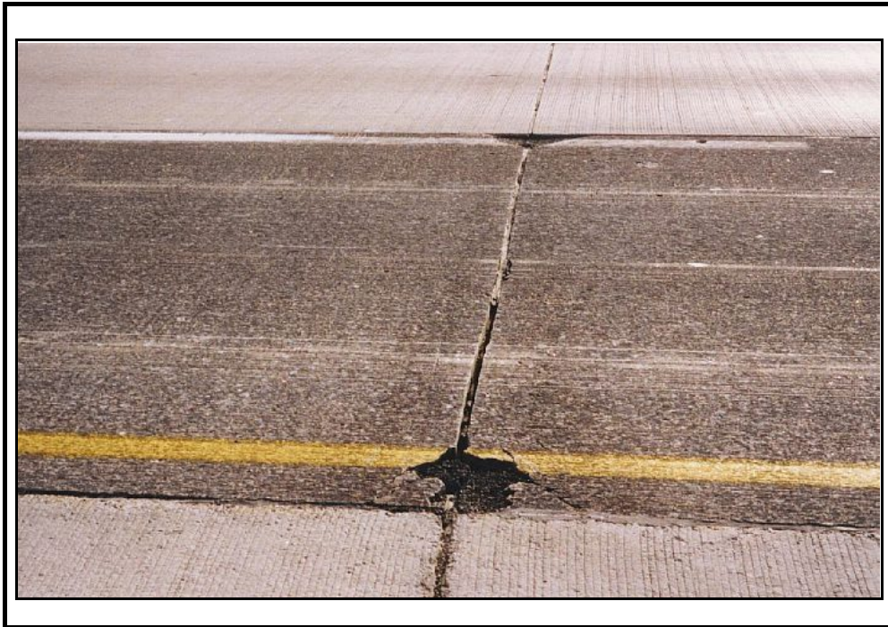
Photo C-15. Joint Sealant Damage in Jointed Concrete Pavement
