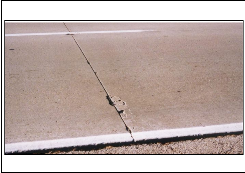
Photo C-12. Transverse Joint Spalling in Jointed Concrete Pavement, Low Severity
