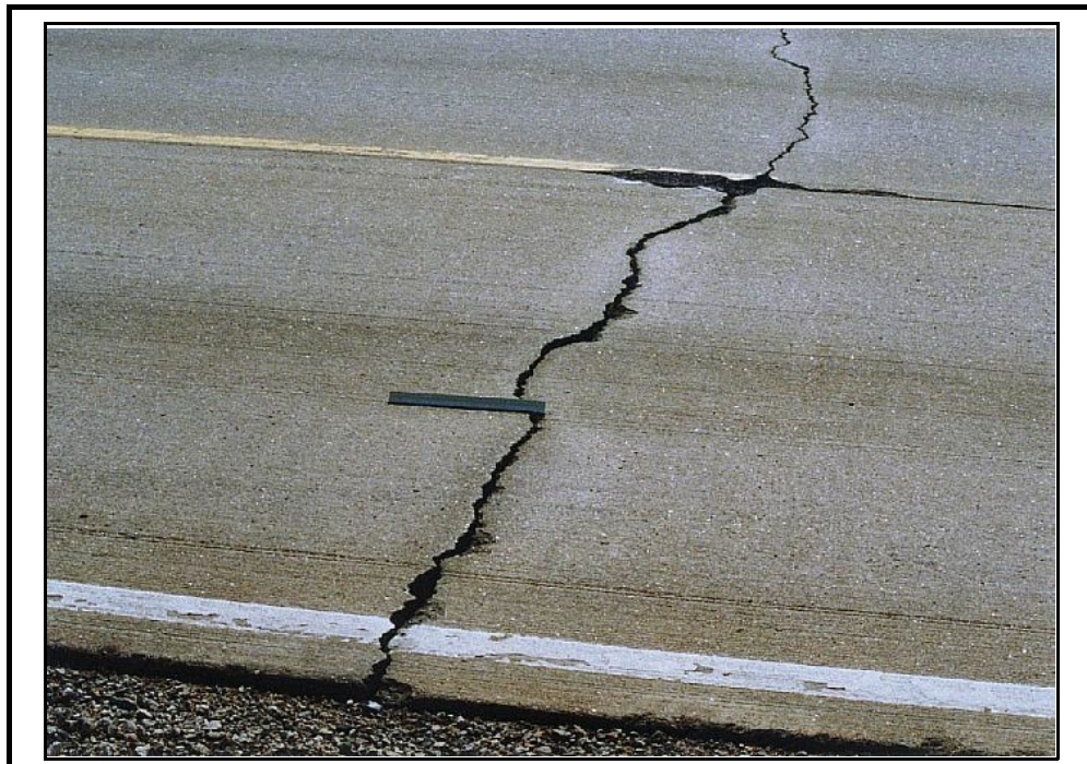
Photo C-10. Faulting in Jointed Concrete Pavement
