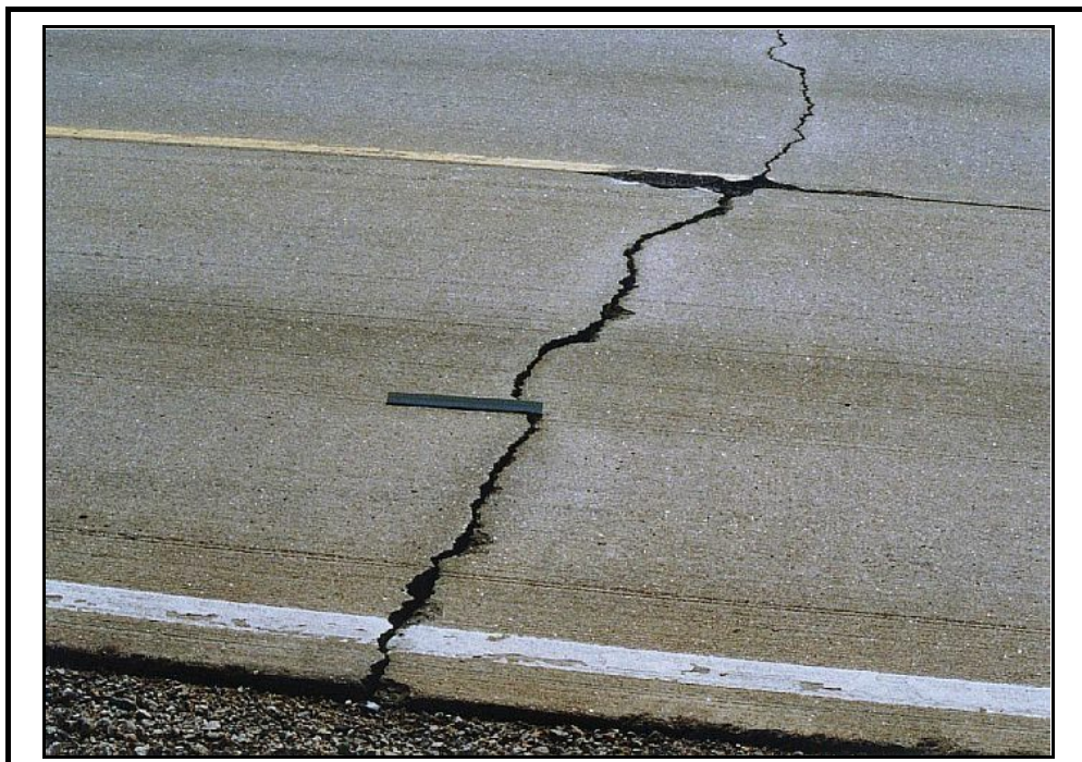
Photo C-19. Transverse Cracking in Jointed Concrete Pavement, High Severity
