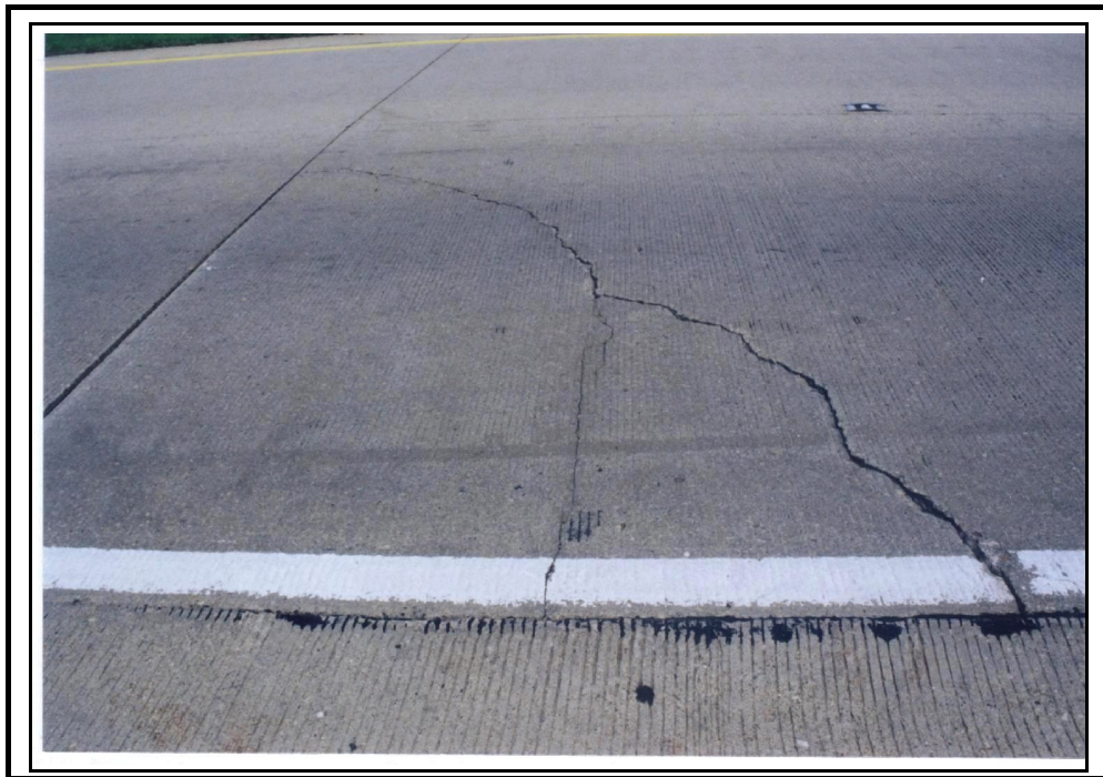
Photo C-23. Corner Breaks in Jointed Concrete Pavement, High Severity
