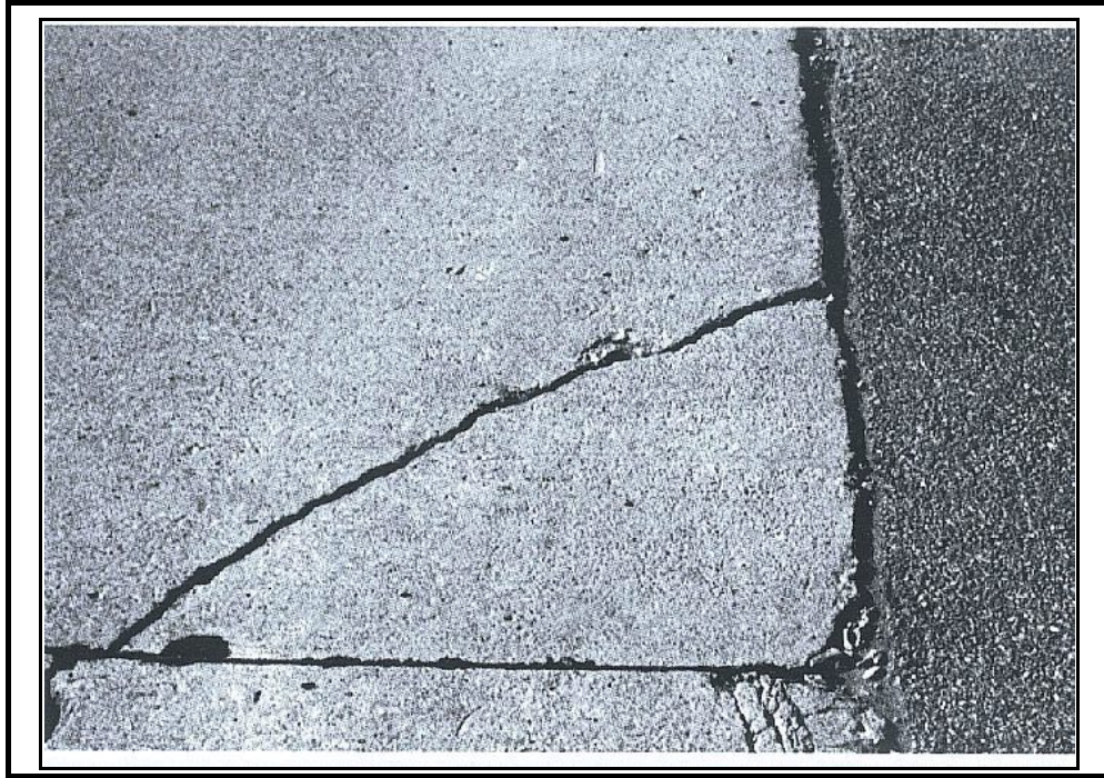
Photo C-22. Corner Break in Jointed Concrete Pavement, Medium Severity
