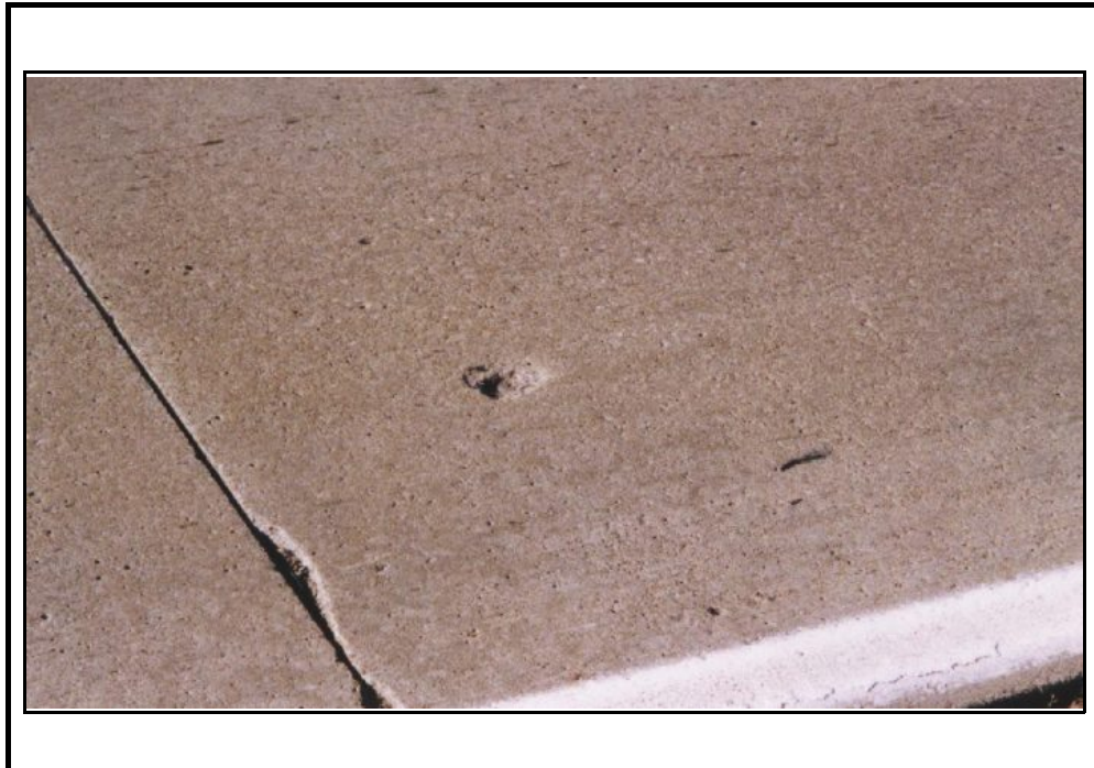
Photo C-4. Popouts in a Jointed Concrete Pavement
