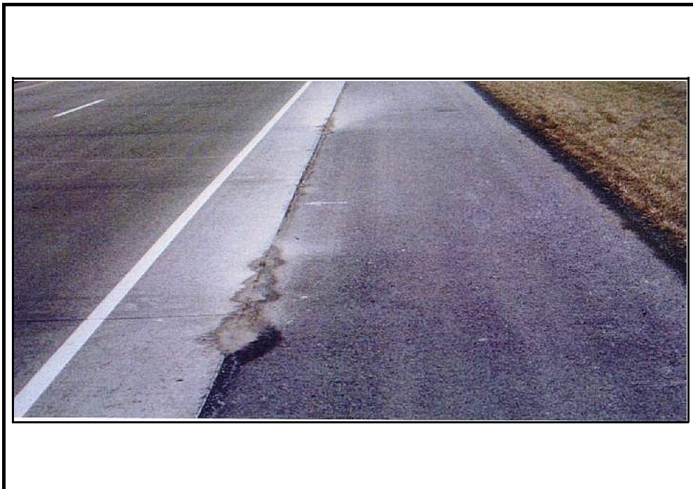
Photo C-8. Pumping in Jointed Concrete Pavement, Low Severity
