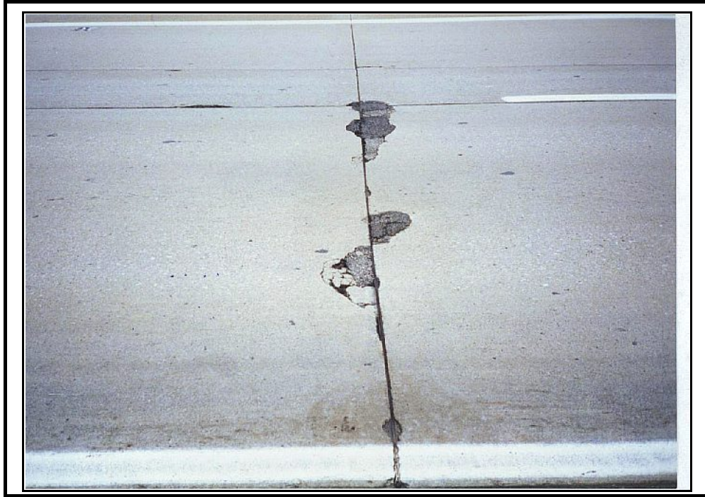
Photo C-5. Patching in Jointed Concrete Pavement, Low Severity
