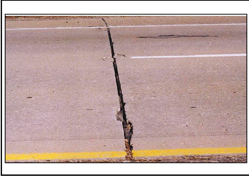
Photo C-14. Joint Sealant Damage in Jointed Concrete Pavement
