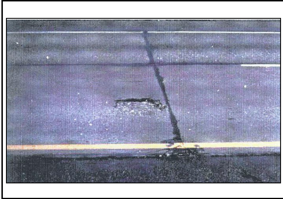
Photo C-16. Pressure Damage in Jointed Concrete Pavement
