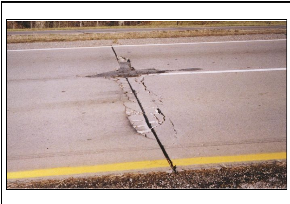
Photo C-13. Transverse Joint Spalling in Jointed Concrete Pavement, High Severity
