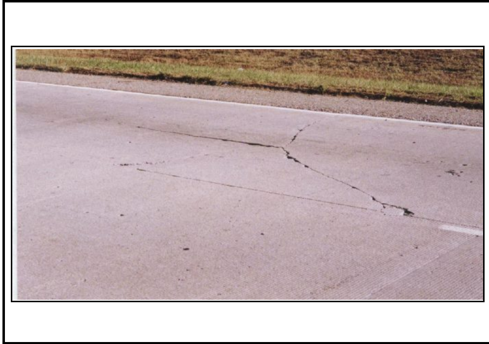
Photo C-20. Longitudinal Cracking in Jointed Concrete Pavement, Medium Severity
