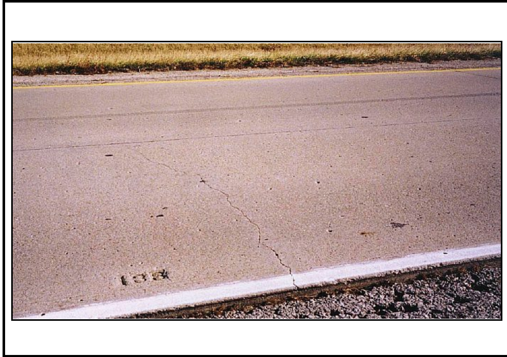
Photo C-18. Transverse Cracking in Jointed Concrete Pavement, Low Severity
