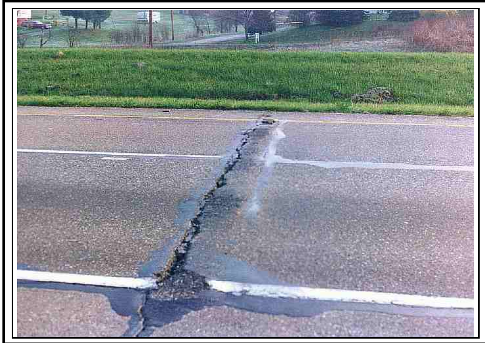
Photo B- 20. Pressure Damage/Upheaval in Composite Pavement, Medium Severity
