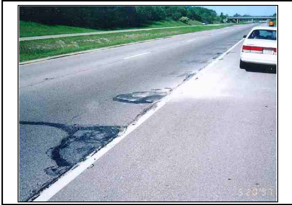
Photo B-11. Pumping in Composite Pavement, Medium Severity
