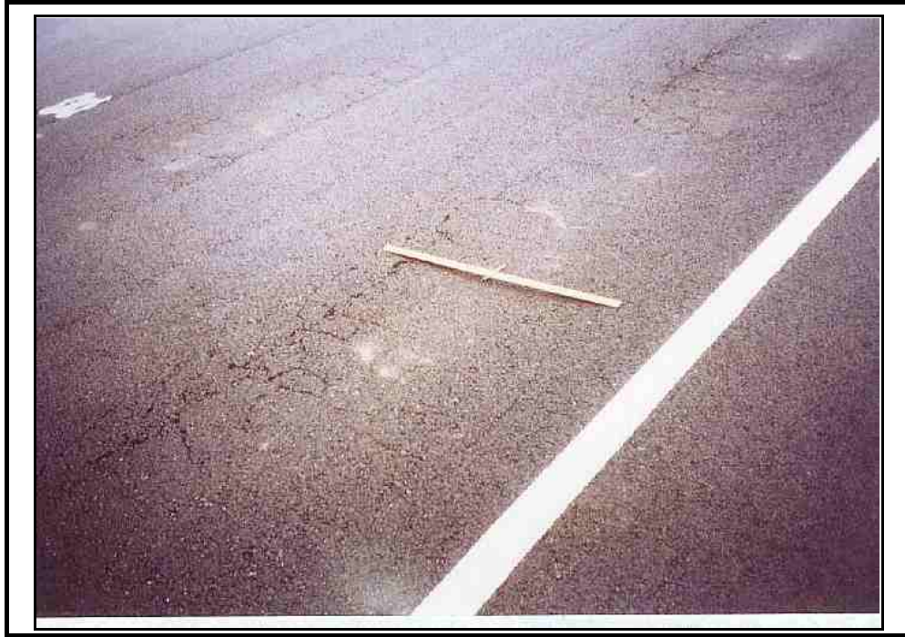
Photo B-9. Rutting, Medium Severity
