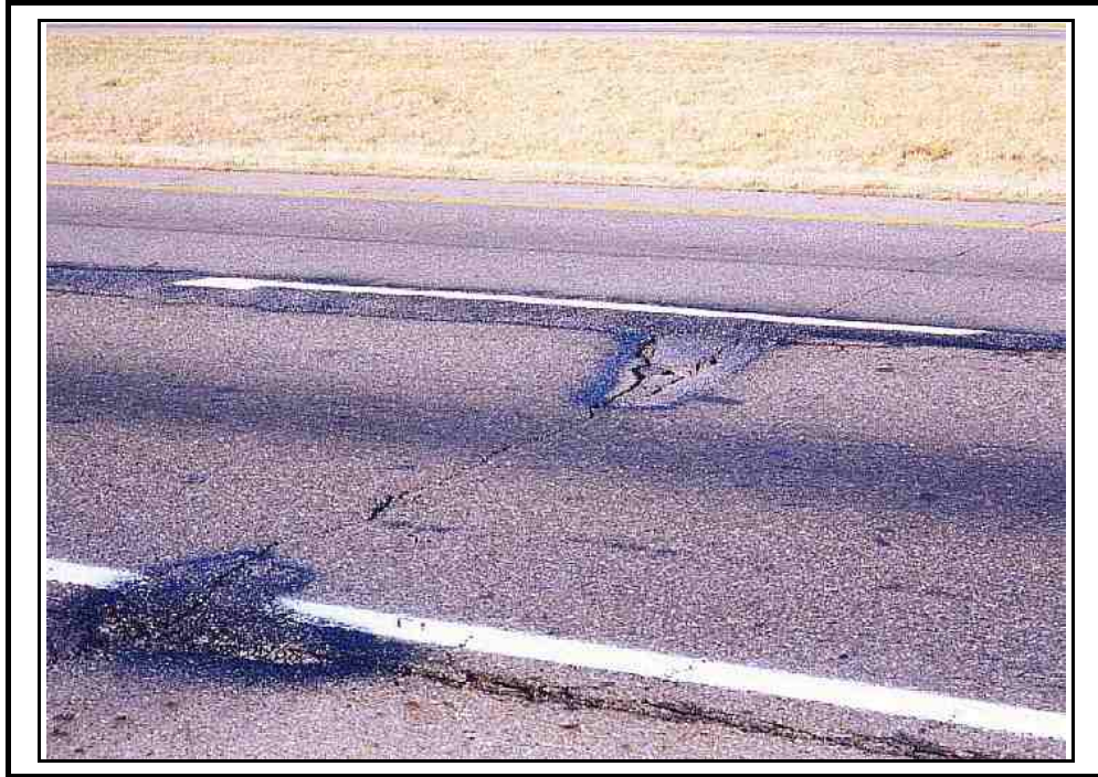
Photo B- 17. Jointed Base, Reflection Cracking in Composite Pavement, Medium Severity
