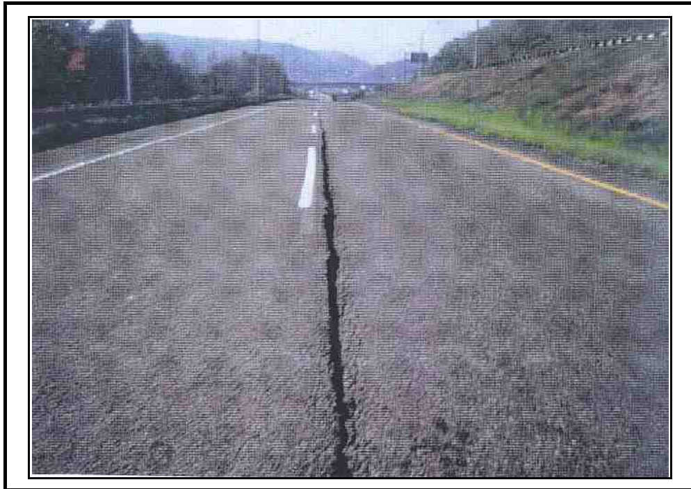
Photo B- 19. Longitudinal Cracking in Composite Pavement, High Severity
