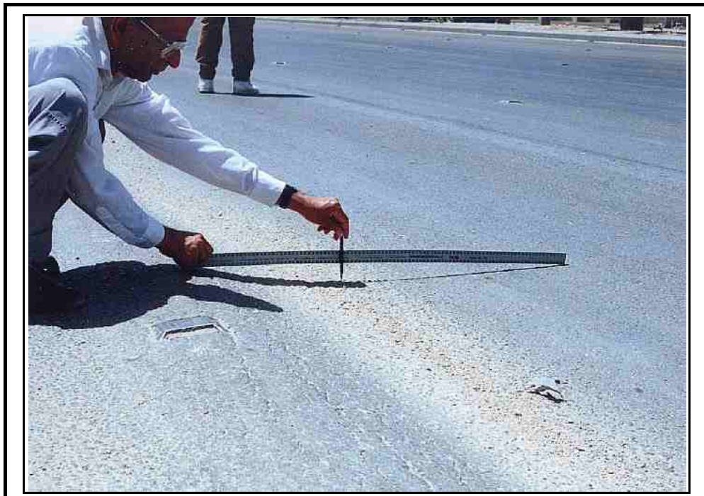
Photo B-10. Rutting, High Severity
