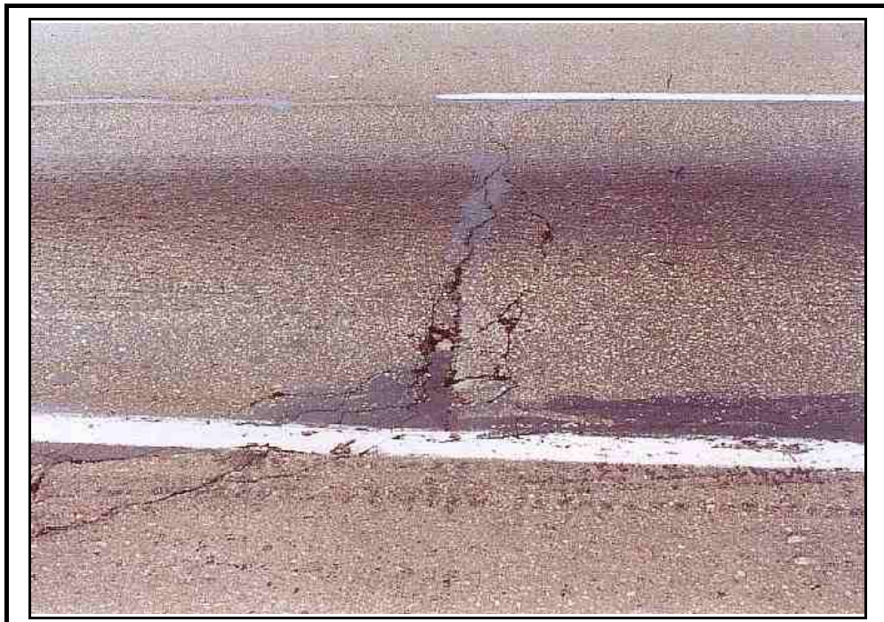
Photo B-22. Crack Sealing Deficiency, Cracks not sealed properly
