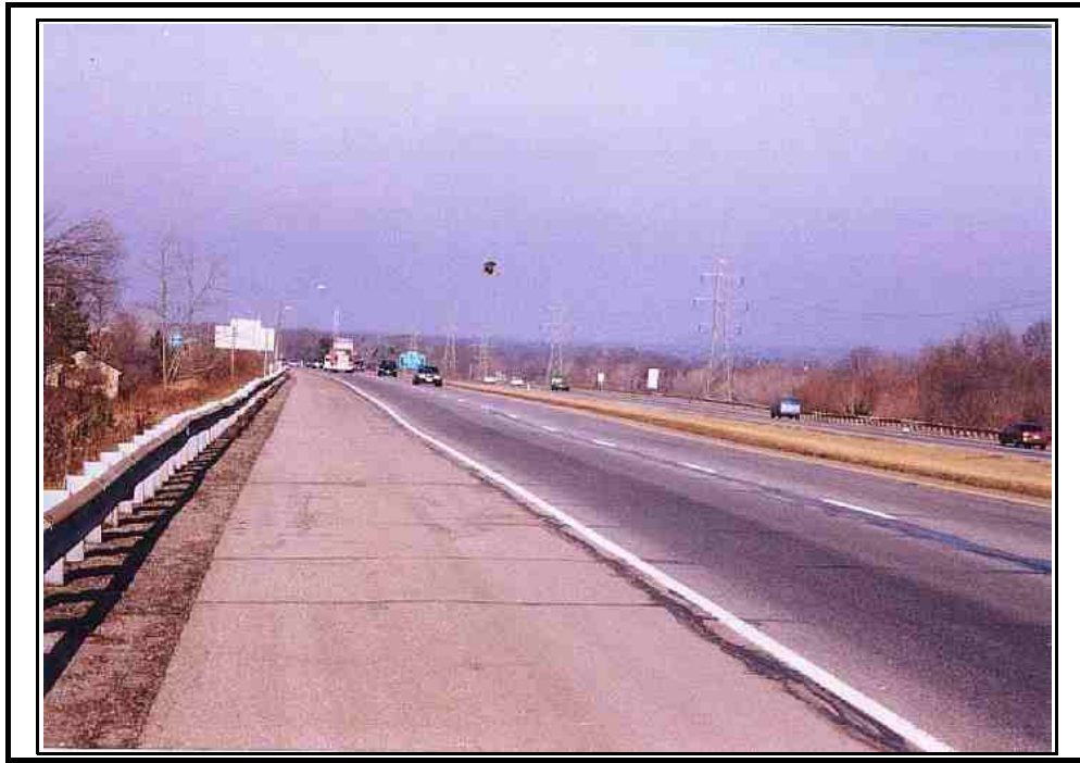
Photo B-14. Settlement in Composite Pavement, Medium Severity
