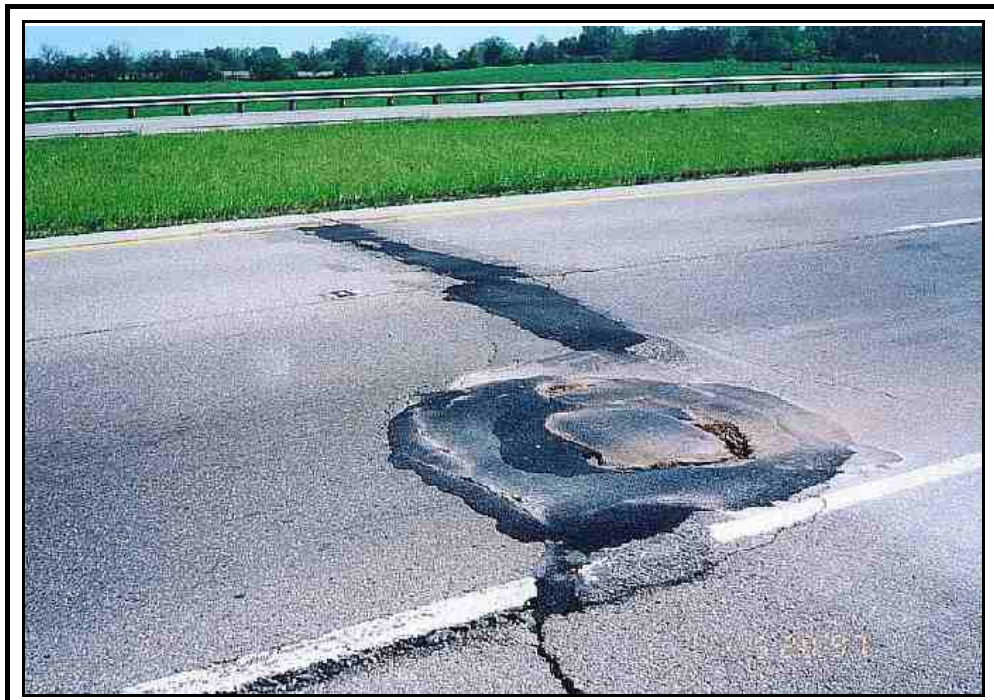
Photo B-12. Pumping in Composite Pavement, High Severity
