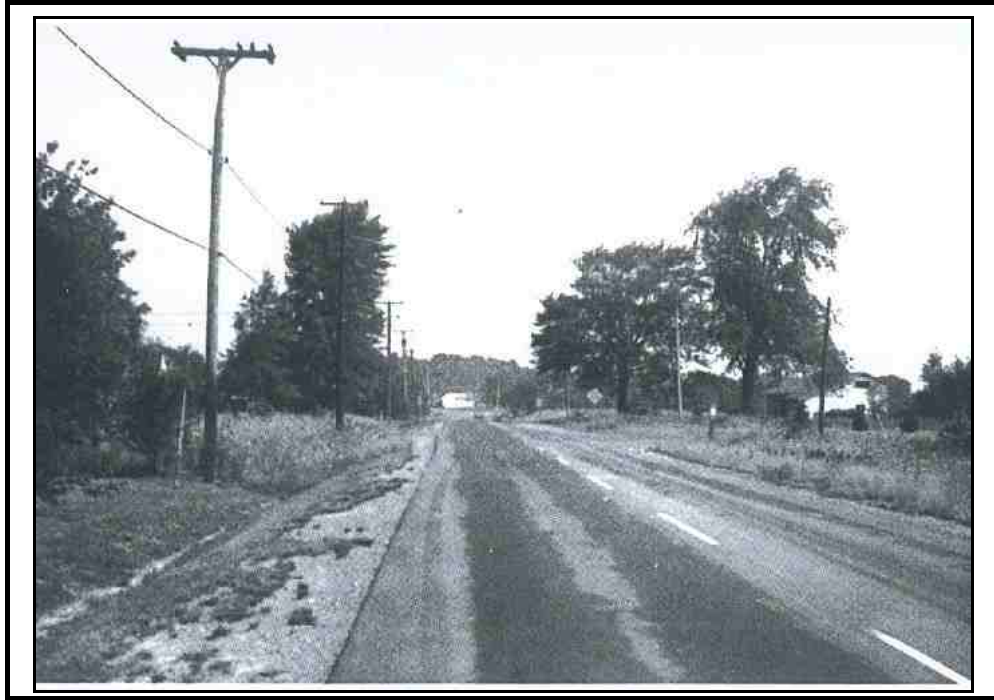
Photo B-3. Bleeding, High Severity
