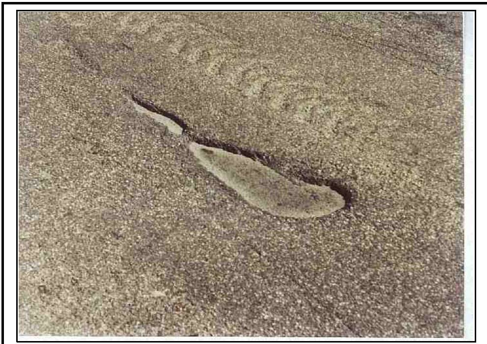
Photo B-8. Debonding in Composite Pavement, Medium Severity
