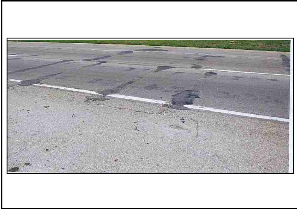
Photo B-5. Patching in Composite Pavement, Medium Severity
