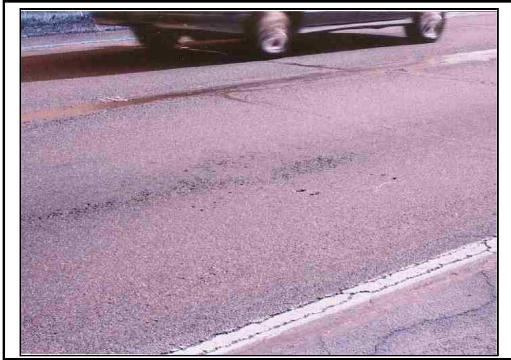
Photo B-1. Raveling in Composite Pavement, Medium Severity
