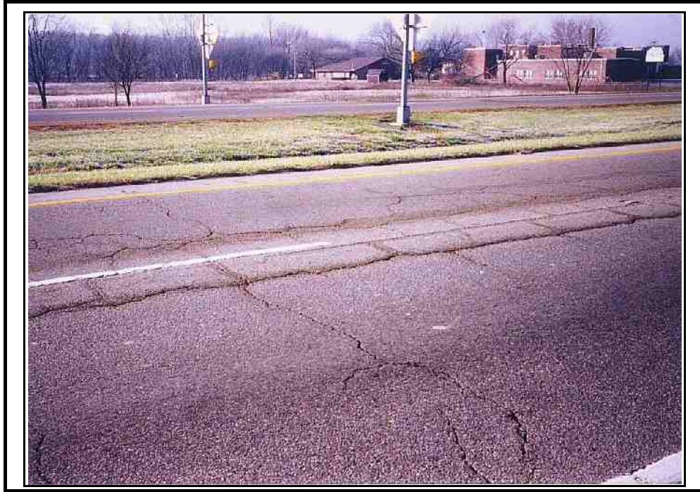
Photo B-21. Crack Sealing Deficiency, Unsealed Cracks
