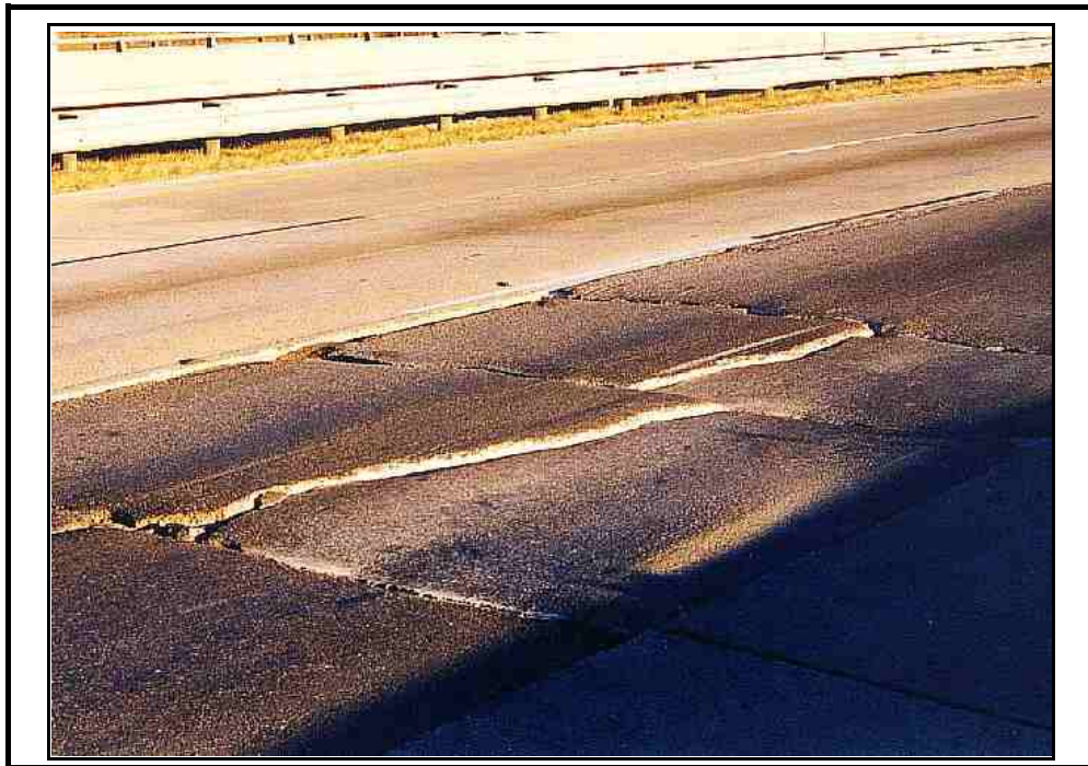
Photo B-13. Shattered Slab of Composite Pavement, High Severity
