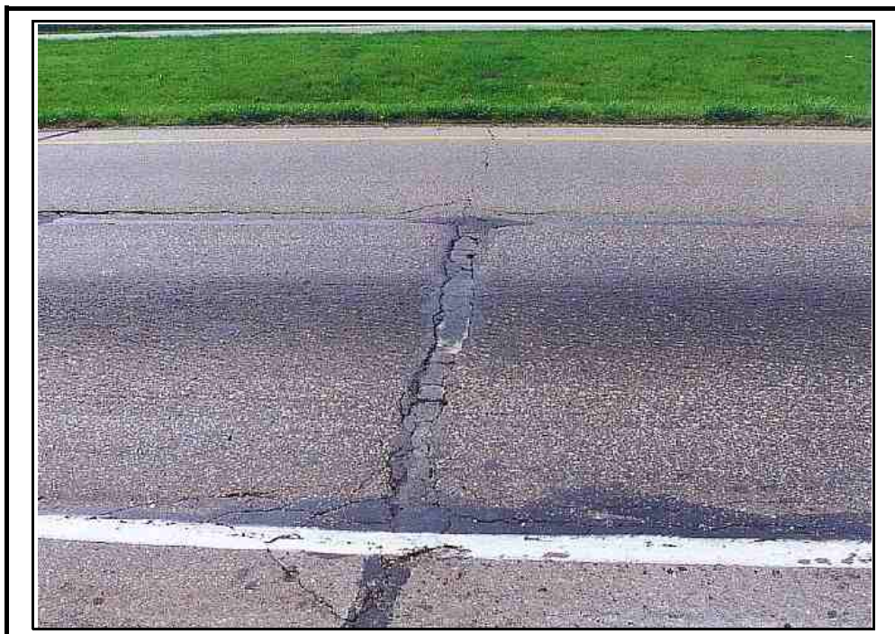
Photo B- 18. Jointed Base, Reflection Cracking in Composite Pavement, High Severity
