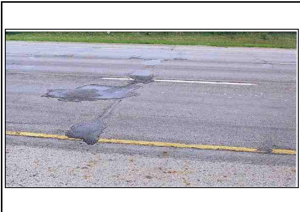
Photo B-6. Patching in Composite Pavement, High Severity
