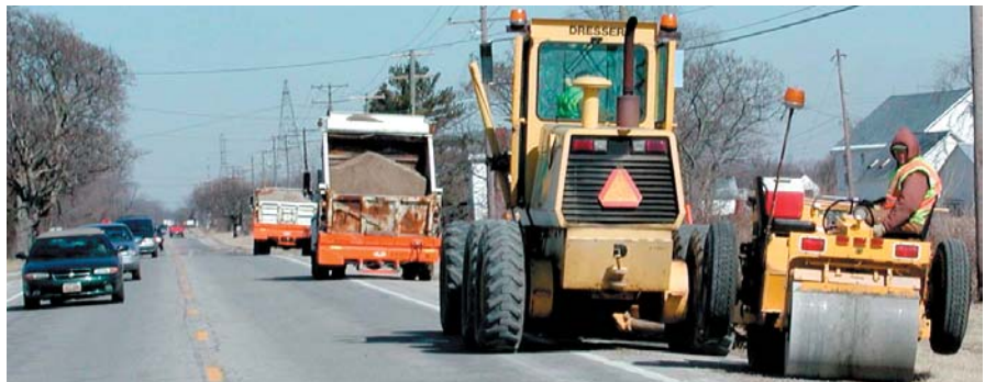
Consistent maintenance activities, such as this berm replacement being conducted by District 6 forces on U.S. Route 62 in southern Franklin County, have significantly improved Ohio's pavement conditions.
