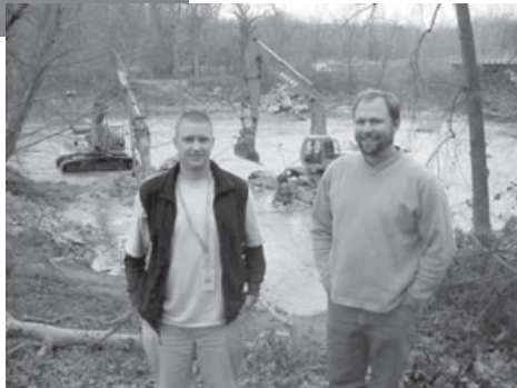
OES Waterway Permits Supervisor Mike Pettegrew and Environmental Specialist Don Rostofer on site during the St. Johns Dam removal on the Sandusky River.
