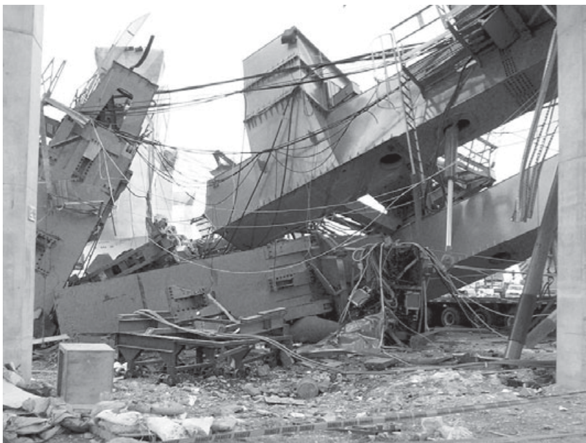
The collapsed truss stopped work on the Maumee River Crossing main span.
