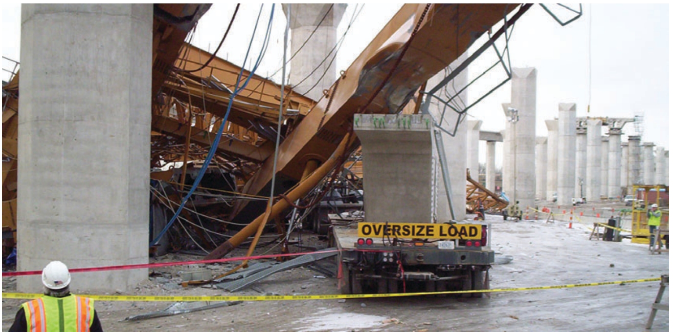
Workers survey the twisted aftermath of the collapsed erection truss on Toledo's Maumee River Crossing project.
