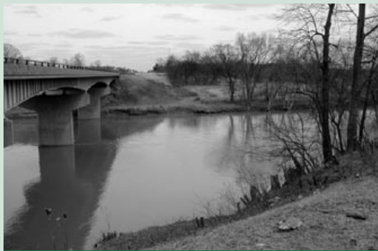
Clearing work has begun next to the existing U.S. Route 24 bridge over the Tiffin River, which will be replaced as part of the project.
