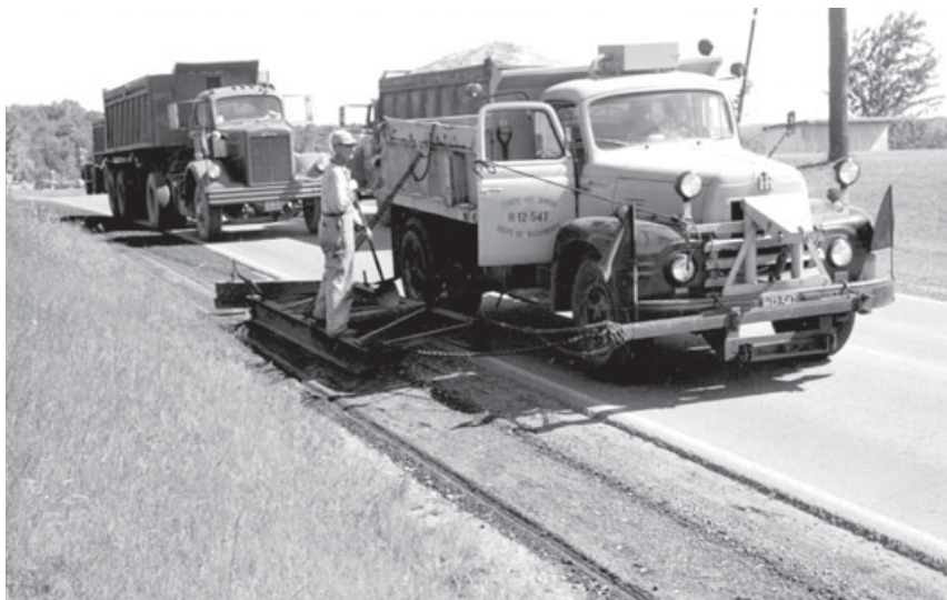
Ohio Department of Highway's workers conduct berm maintenance in the late 1950s on State Route 44 in Geauga County.
