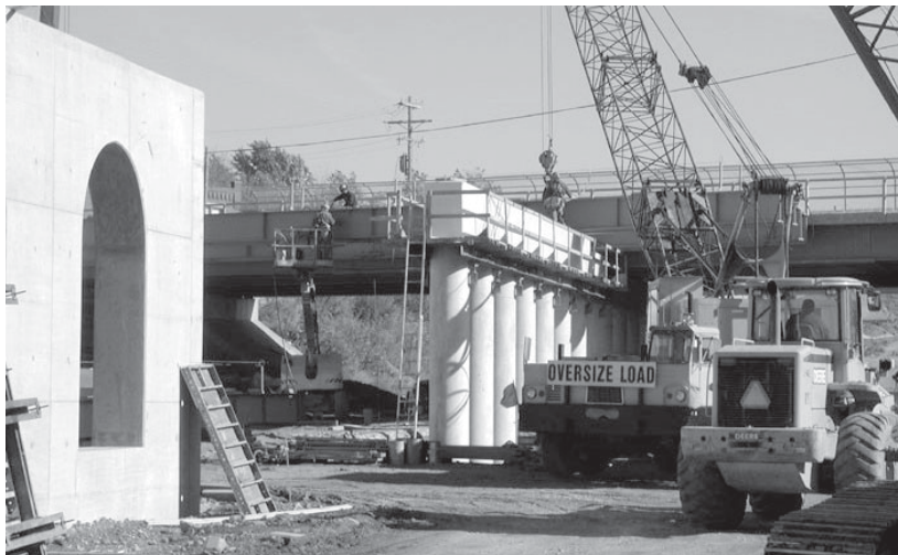
Heavy machinery secures a bridge column for the High Street Cap in downtown Columbus, part of the Interstate 670 reconstruction project completed in 2003.
