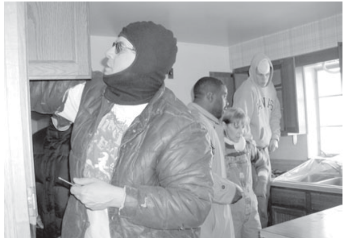
Representatives from Ohio's Habitat for Humanity program salvage items from a house ODOT will demolish for the upcoming Interstate 270/State Route 161/Sunbury Road project in Franklin County.
