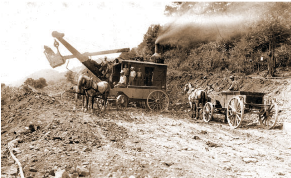
Early 1900s road construction project on Aberdeen Road in Ripley, Brown County.
